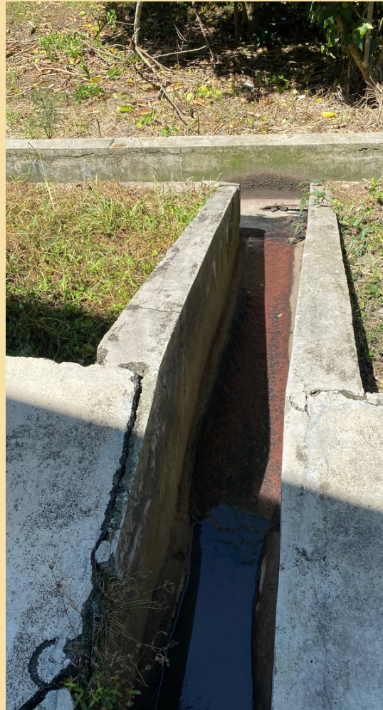
Image 49. Drainage routes towards biogas facility (Source: Photo taken at ATI-ITCPH, 2022)
